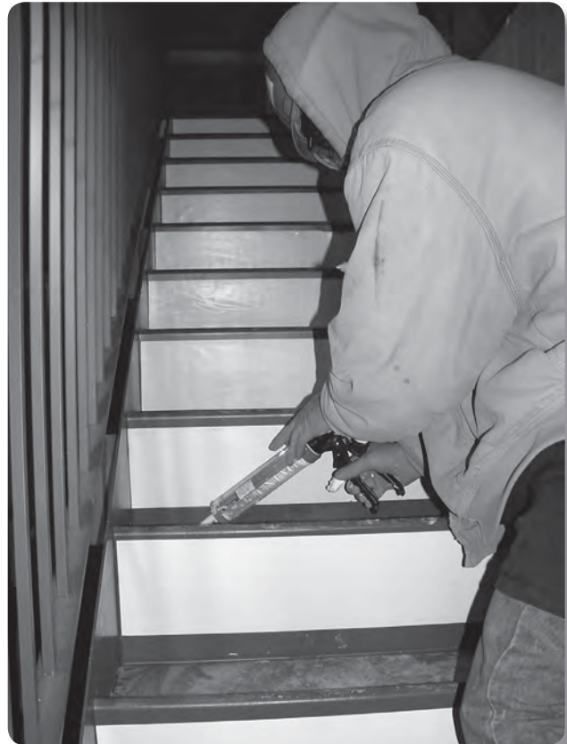
Problem: Manually squeezing caulking gun
