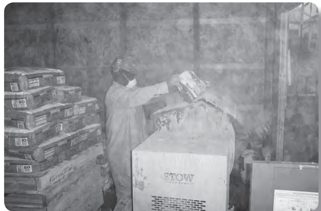
Problem: Traditional method of loading mixer
